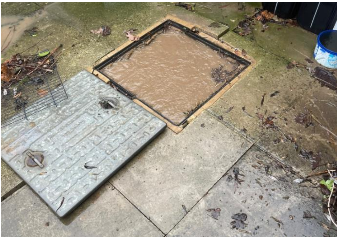
Pic. 3 Flow through manhole 3 at 12:50 2 nd January 2024
