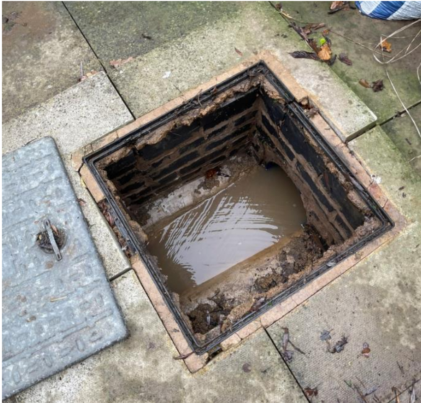
Pic. 2 – Flow through manhole 3 at 8:47 2 nd January 2024.
