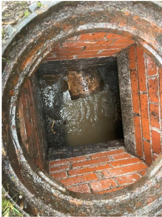
Pic. 6 Manhole 6 with no water flowing through (Note the multiple pieces of broken pipework)
