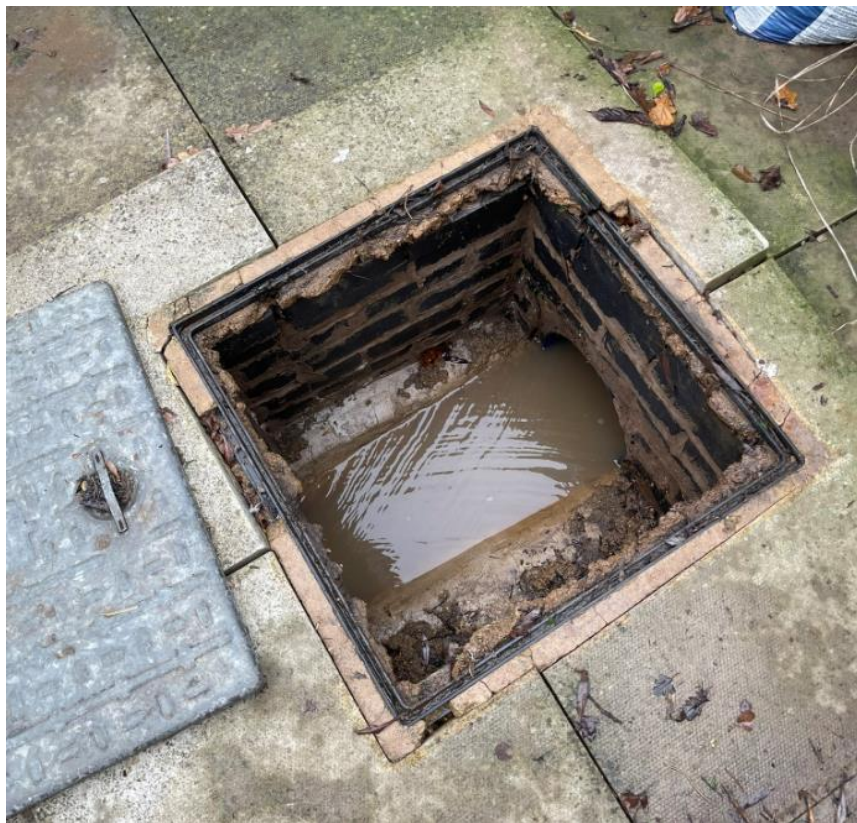
Pic. 2 – Flow through manhole 3 at 8:47 2 nd January 2024.
