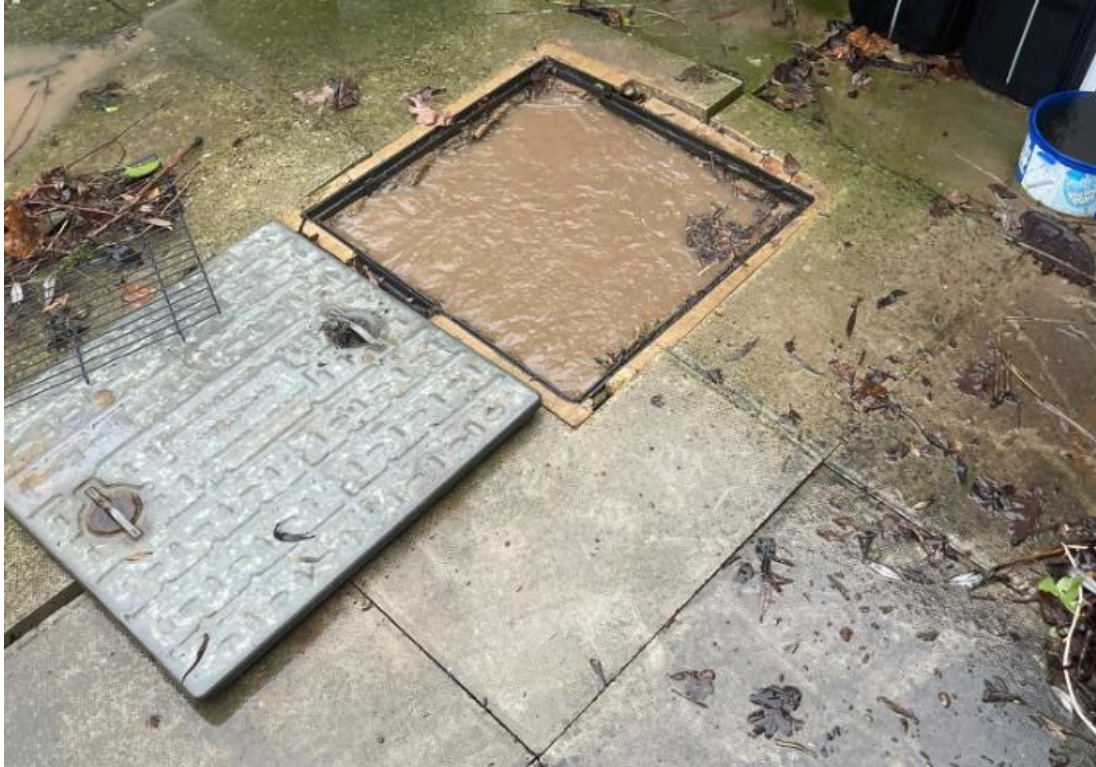
Pic. 3 Flow through manhole 3 at 12:50 2 nd January 2024
