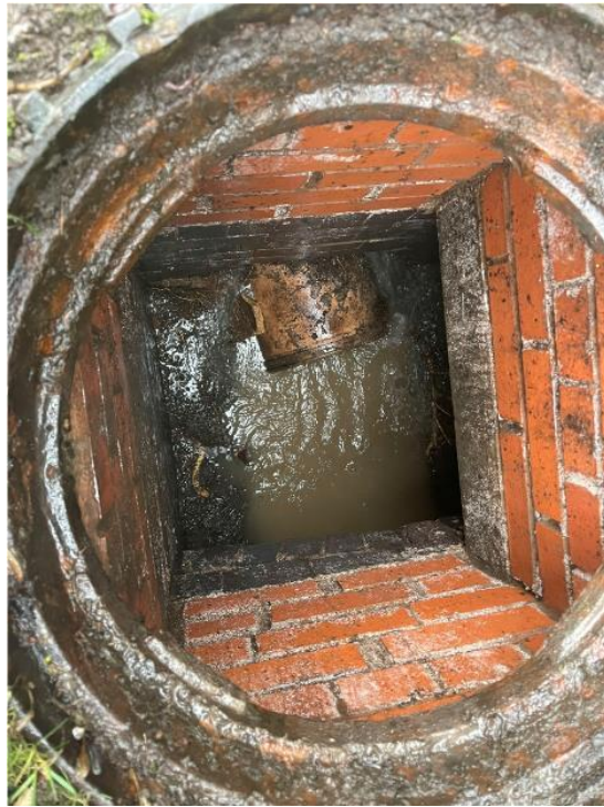
Pic. 6 Manhole 6 with no water flowing through (Note the multiple pieces of broken pipework)
