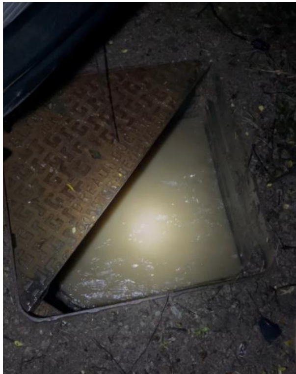
Pic. 7 Manhole 4 full with no indicated water flow
